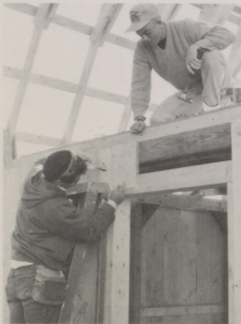
Mr. Shirkey and Corey attach exterior panels as the barn nears completion.
