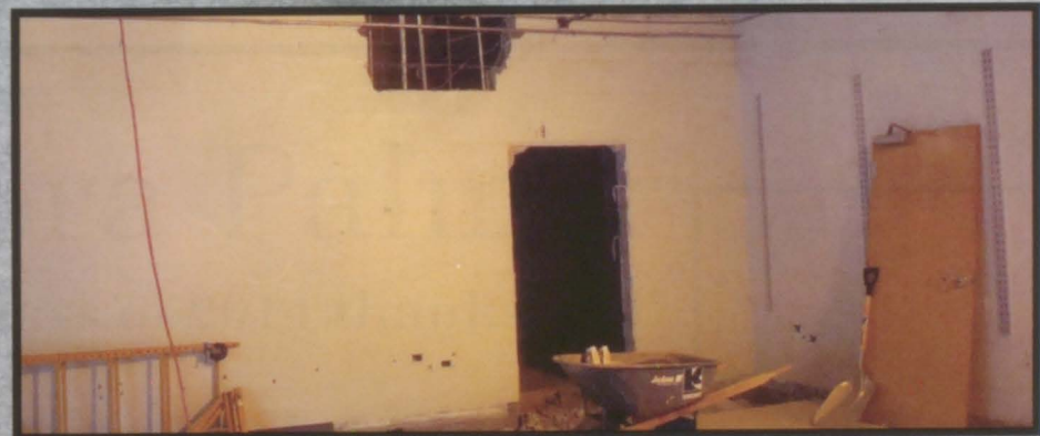
Above, and to the left, is the construction of the new art room.
